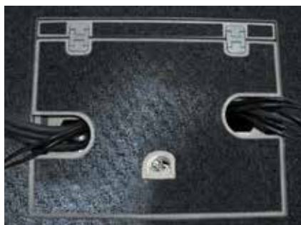
CCBBSCTCAL Cover with cable egress installed with carpet inserts.
